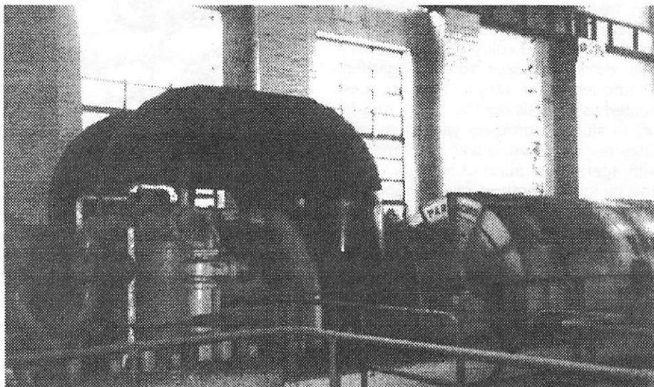
Turbine Generator - White Bay Power Station
