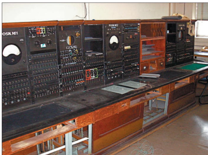
The disused testing desk in the 1957 Balmain Telephone Exchange
