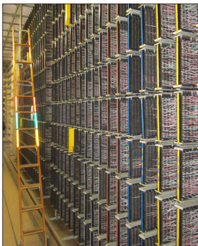
Some of the very colourful wiring that is still in use today. A technician was seen up that ladder several times during the open day.
